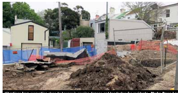
Vibrations from excavation close to houses is causing damage and headaches for residents Photo: Bruce Lay
